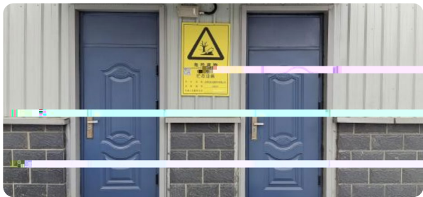
Temporary Storage Room for Hazardous Waste
